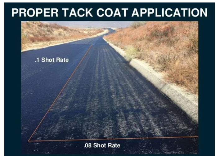
Poor Tack Coat VS Good Tack Coat
